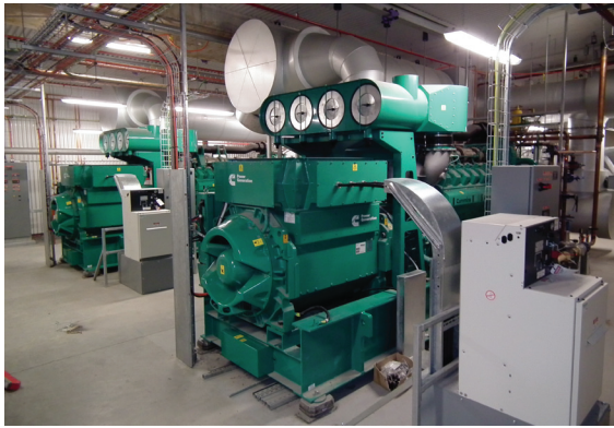
These two 2MW lean-burn gas fueled generator sets are in operation at a cogeneration plant that provides base load power and hot water for an Australian hospital.
