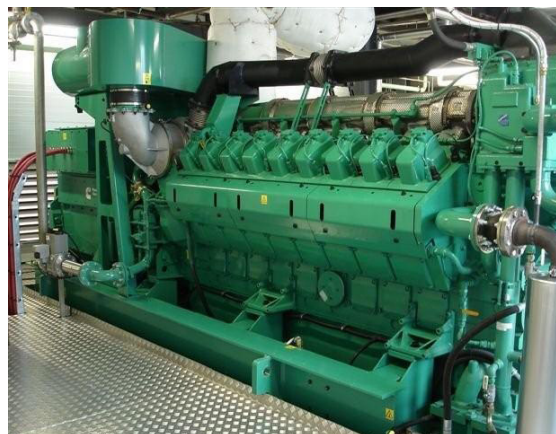
This 2 MW lean-burn gas engine generator set supplies heat, steam and power for a Danish poultry farm, and heat for a nearby village.
