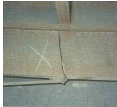
Cracked Frame Member
