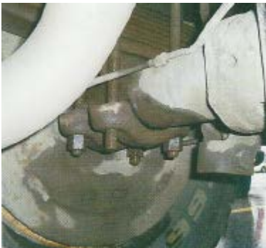
U-Bolt Missing Fastener
